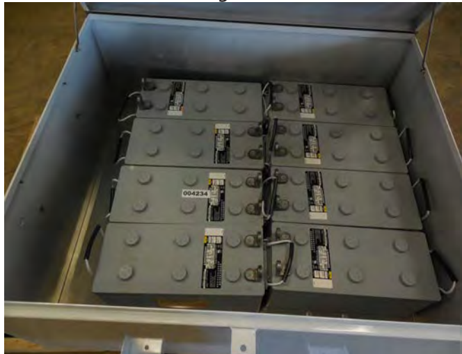
T-8X8D Enclosure with eight 8D batteries
