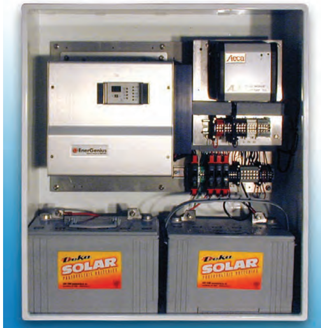
WF2 Enclosure with two G31 batteries
