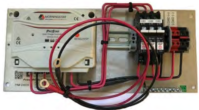
PRE Control Panel with a 30 amp ProStar
