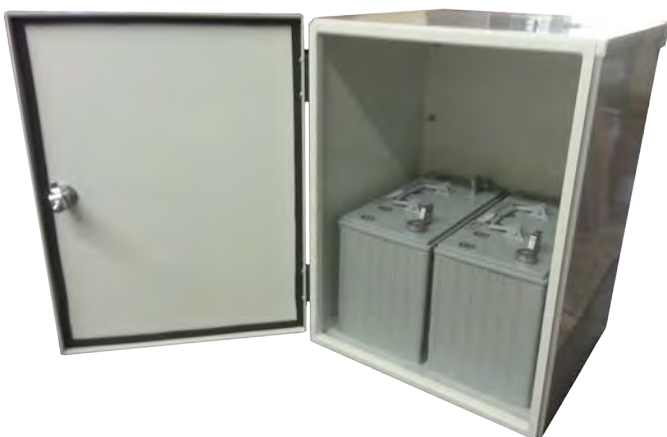
F2 Enclosure with two G31 batteries
