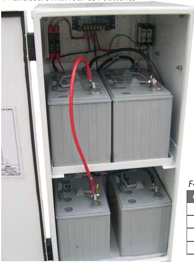
F4 Enclosure with four G31 batteries
