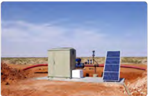
AUTOMATION AND CONTROL
