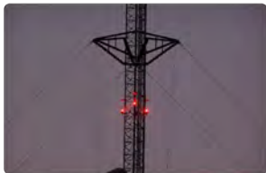
FAA RADIO TOWER LIGHTING
