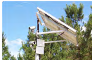
SECURITY AND SURVEILLANCE
