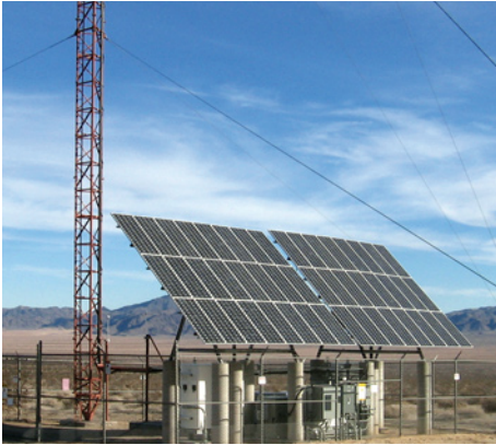
SunWize® Power Station
