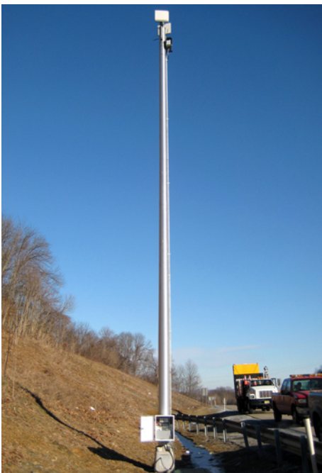
SunWize® Power Online System
