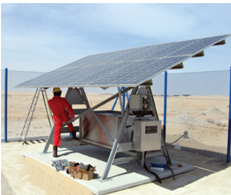
2400 watt SunWize Power Station, cathodic protection
