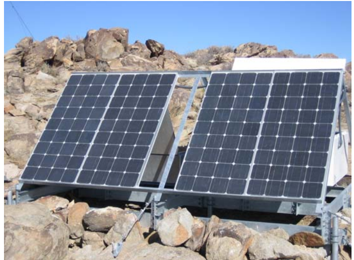
Example of SunWize system installed in a rocky location requiring special logistical considerations.
