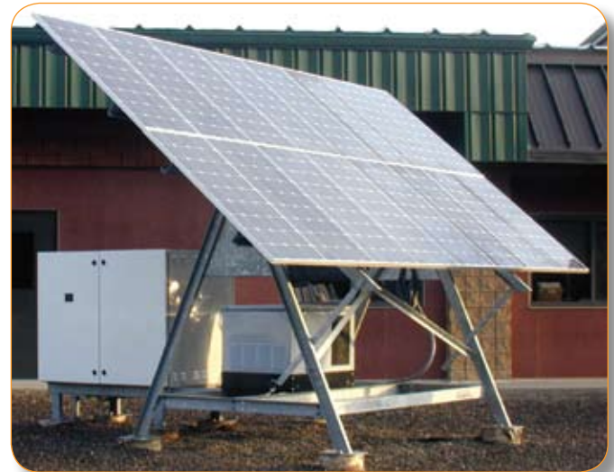
SunWize Power Station
