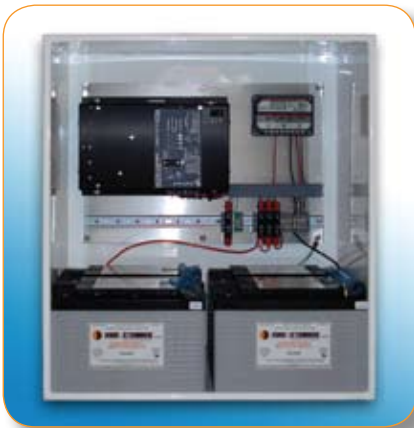
600 watt Power Online System with 48 Vdc, 120AH VRLA batteries, and custom system options
